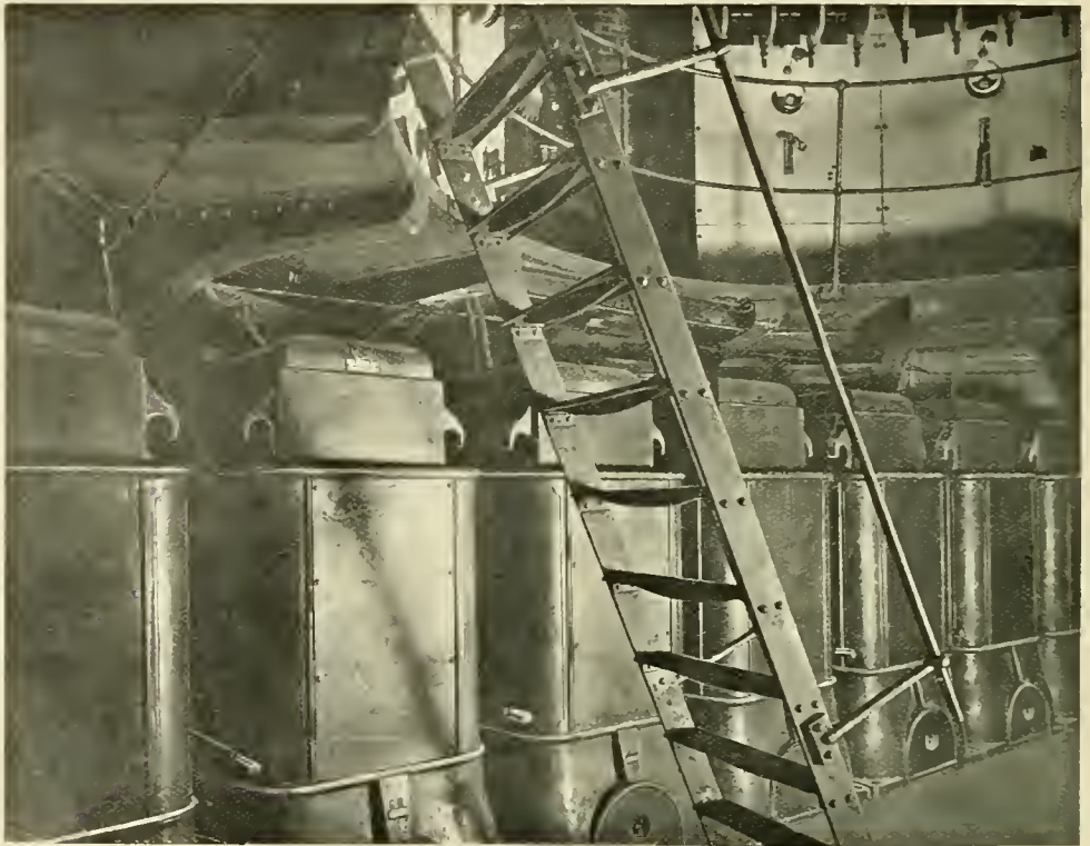
Fig. 185. CENTRAL LONDON RAILWAY: NOTTING HILL GATE SUB-STATION. BANK OF 300-K.W. TRANSFORMERS.
