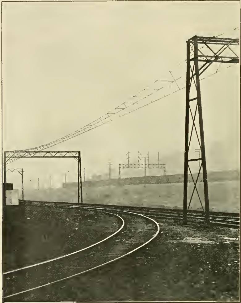
Fig. 224. PHOTOGRAPH SHOWING DOUBLE CABLE SUSPENSION SUPPORTED FROM GANTRIES CONSTRUCTED BY THE WESTINGHOUSE COMPANY.
